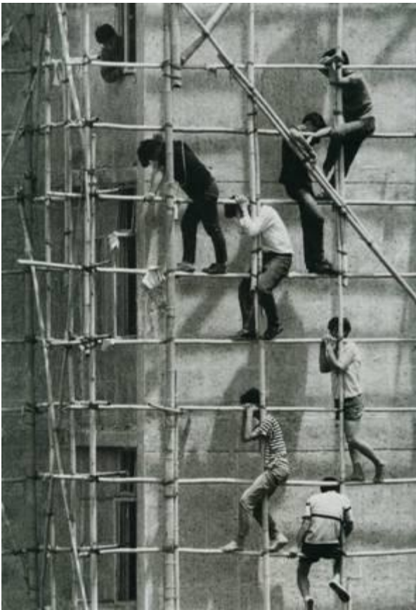
Illegal construction workers
